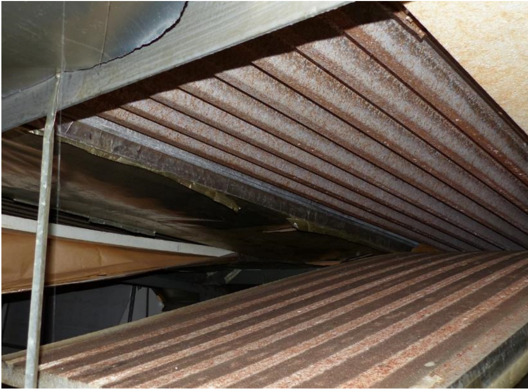
Photograph 11: Corrosion to underside of the aluminium roof cladding. The orange staining is the adhesive for the polystyrene insulation that has become de-bonded.
