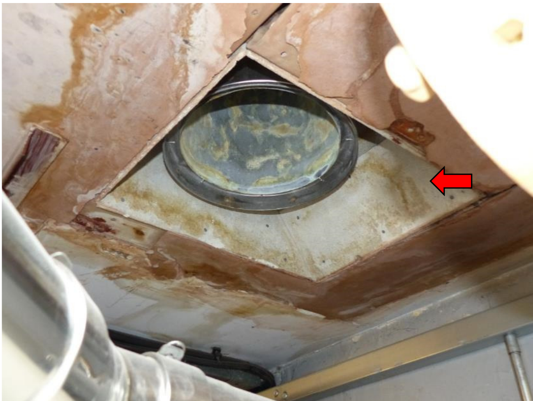
Photograph 24: Cementitious board lining a flue opening to the boiler room roof.
