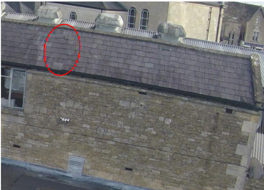
Photograph 22: Slipped slate to the rear of the three storey section.
