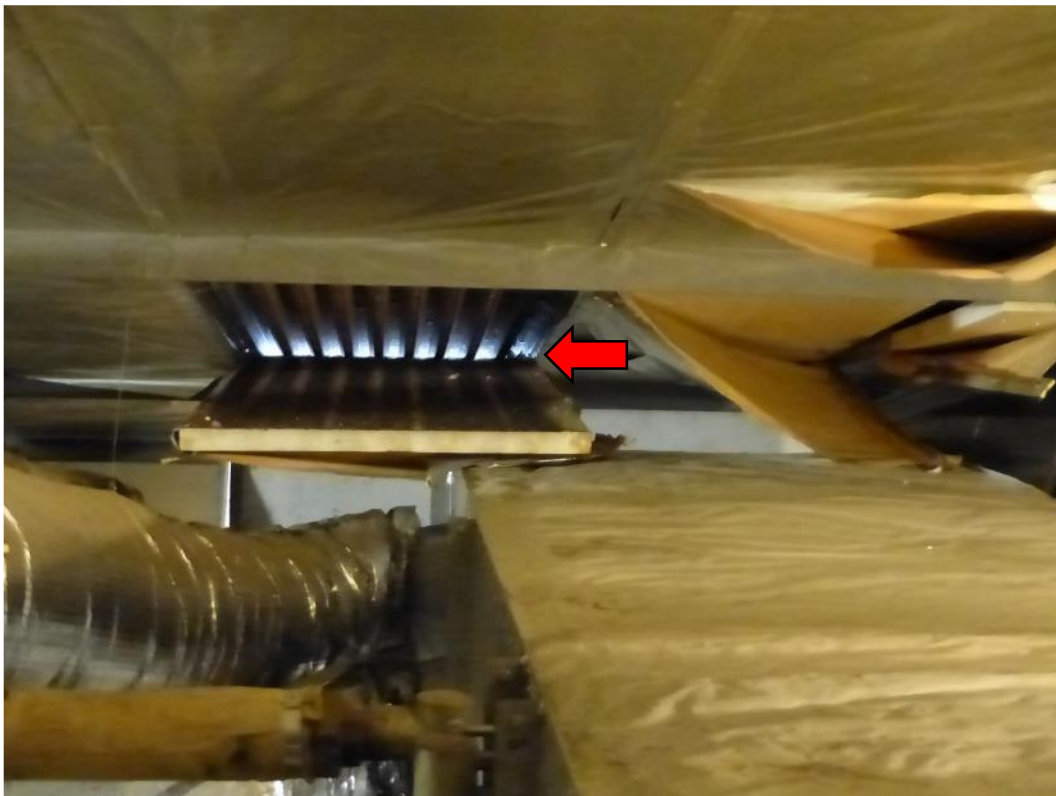
Photograph 12: Light entering the roof void at the exposed knee joint of the main hall mansard roof.
