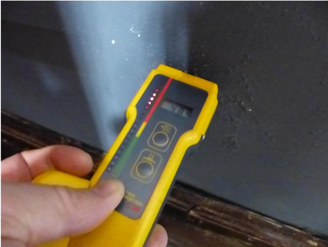
Photograph 37: Dampness to the left hand side of the rear wall of the main hall at low level.
