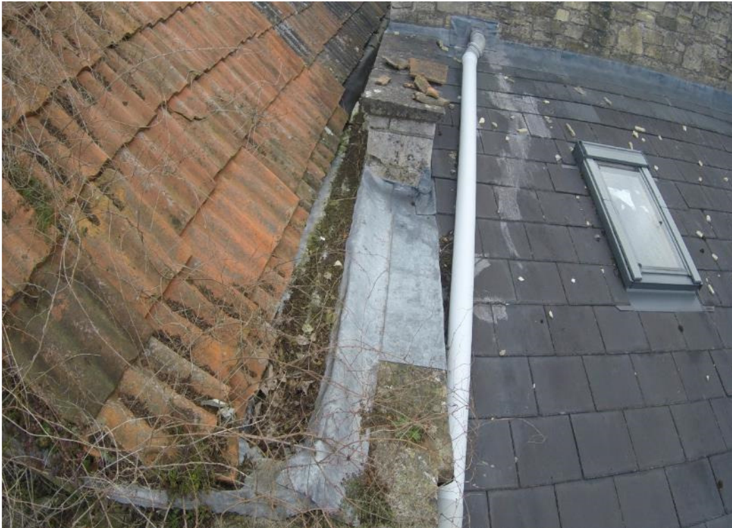
Photograph 27: Blocked gutter to the rear right hand adjoining property.
