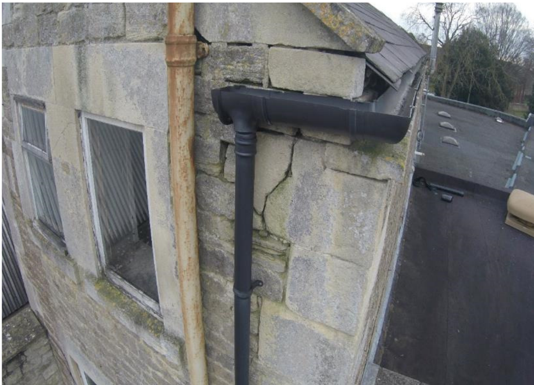
Photograph 36: Cracking and poor pointing to the rear right hand corner of the three storey section.
