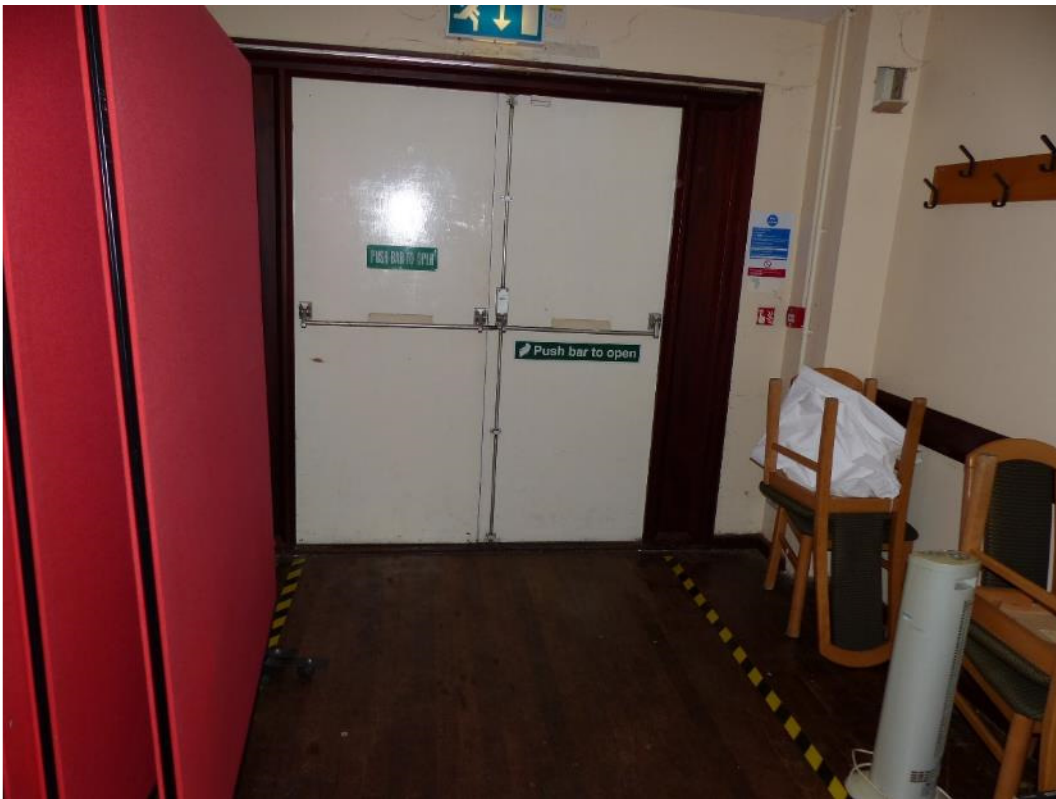
Photograph 39: Combustible items stored in the rear left hand fire escape corridor.
