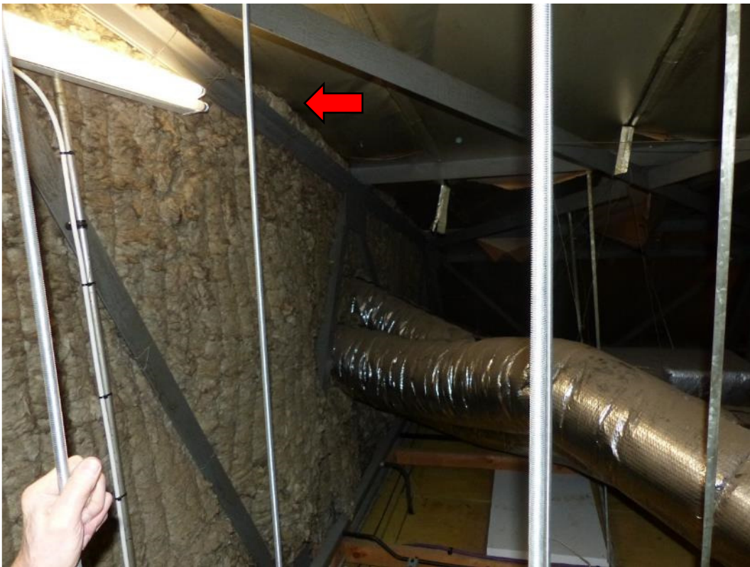
Photograph 15: Fire barrier apparently fixed below the polystyrene insulation and no obvious dampers to the ducts passing through it.
