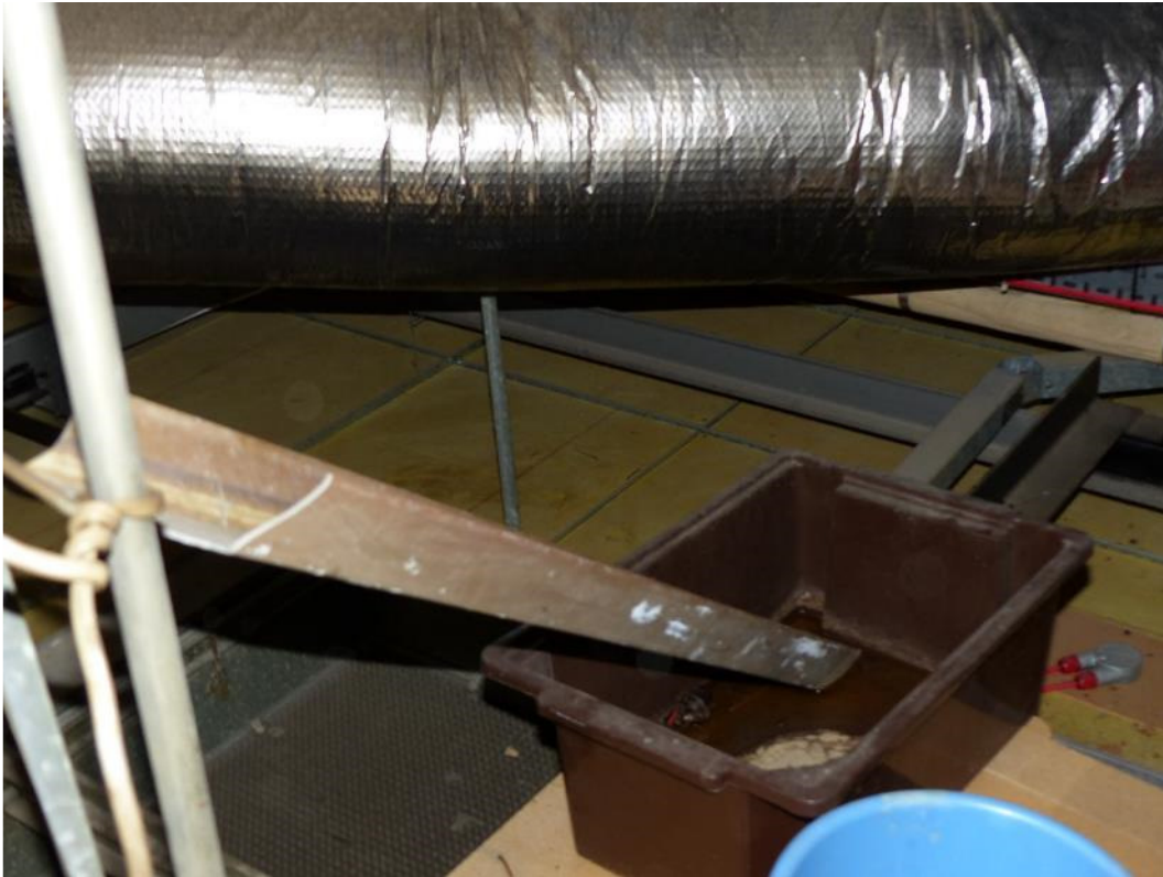
Photograph 13: Makeshift gutter and bucket collecting water from roof leaks over the main hall.
