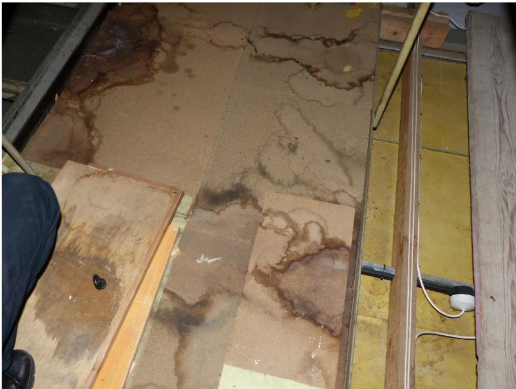
Photograph 14: Water stained boarding to the roof void walkway and additional boards represent a trip hazard.
