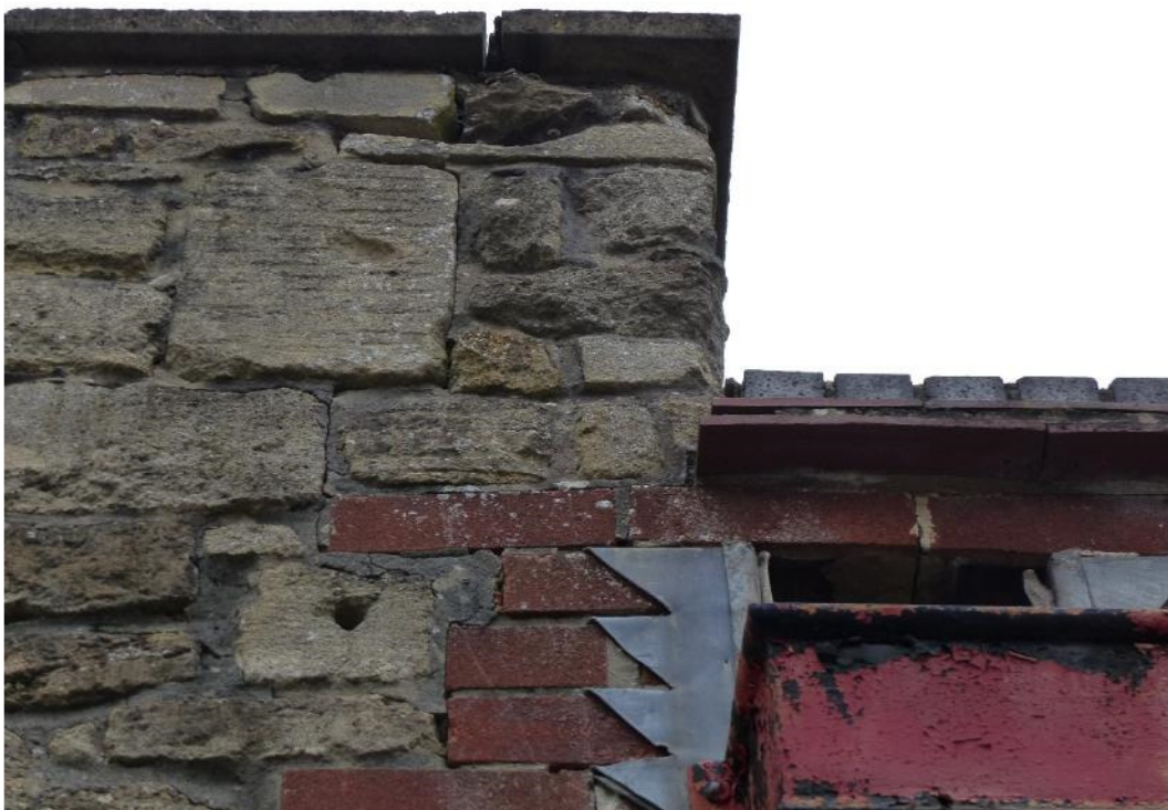
Photograph 30: Differential movement between the main hall and the front extensions to the left hand elevation.
