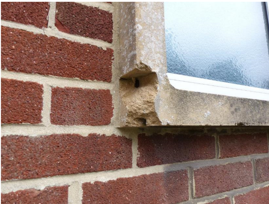
Photograph 34: Spalling to the front window surrounds
