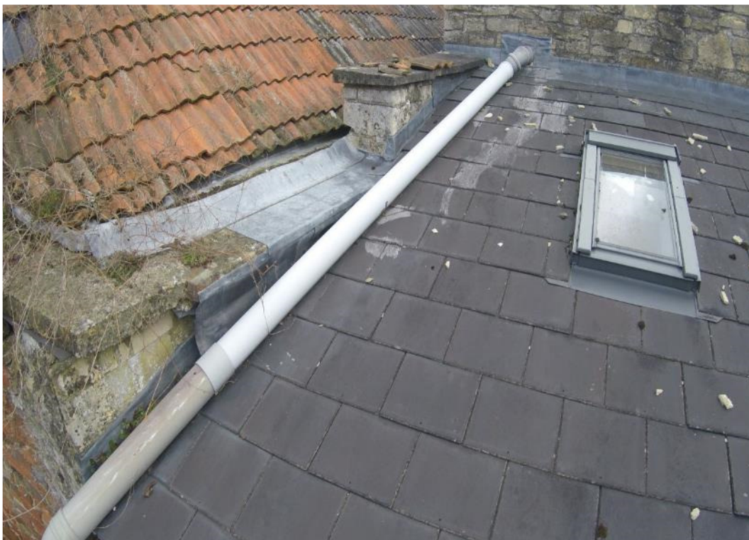
Photograph 26: Flashings to the roof over the laundry room.
