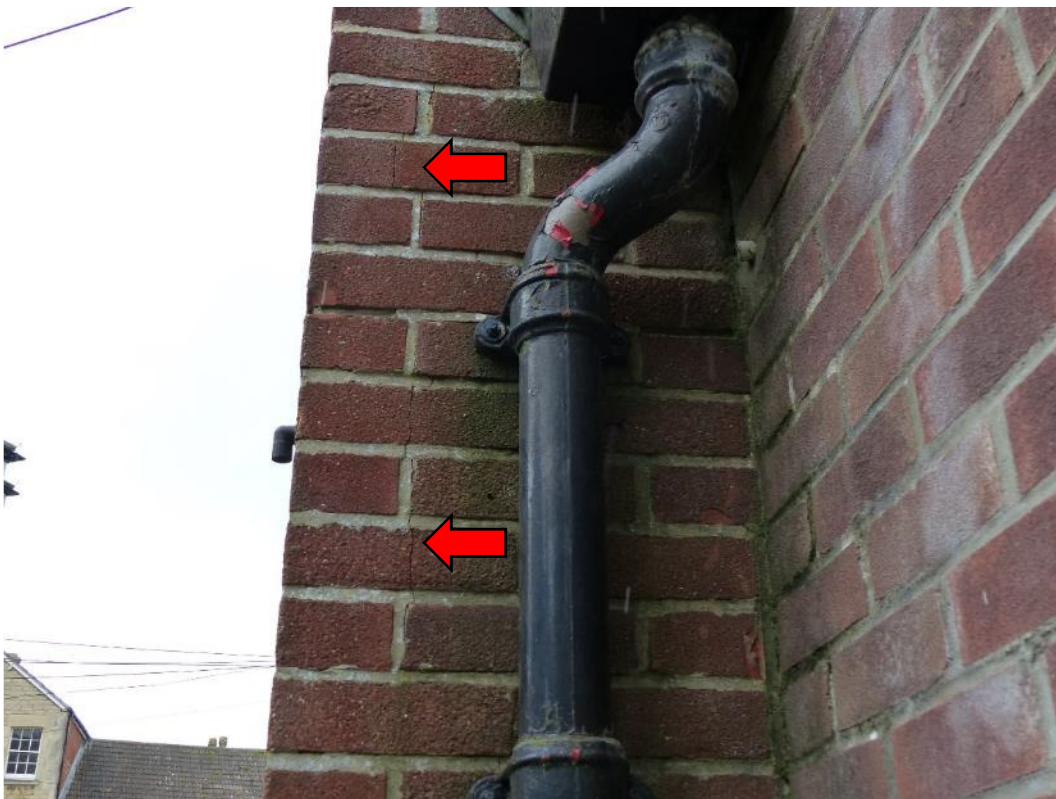
Photograph 32: Cracking to the set-back on the front elevation due to expansion of the brickwork.
