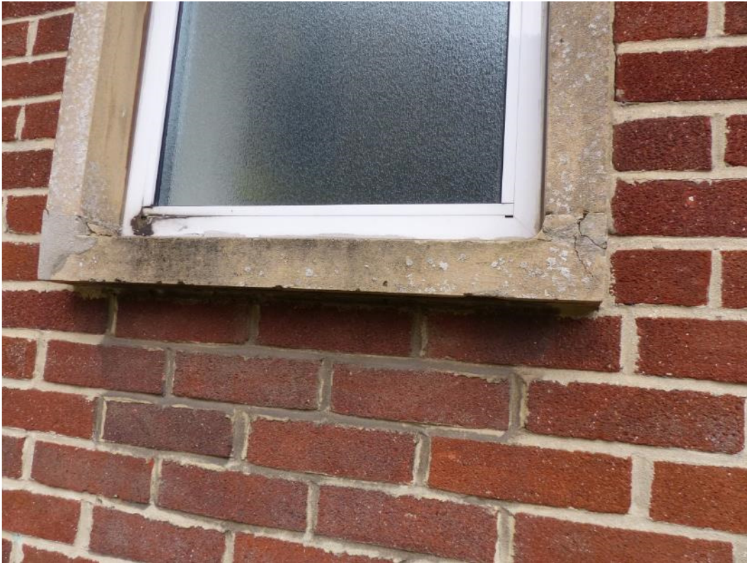
Photograph 33: Cracking and patch repairs to the corners of the front window surrounds.
