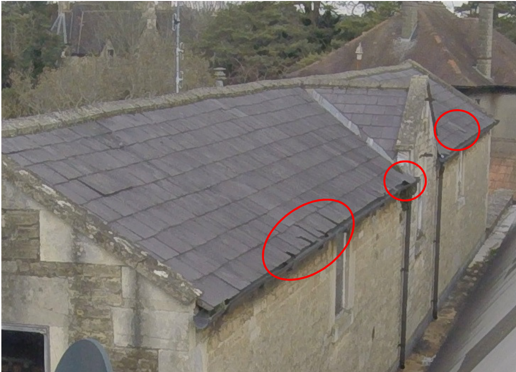
Photograph 21: Slipped and damaged slates to the front roof slopes three storey section.
