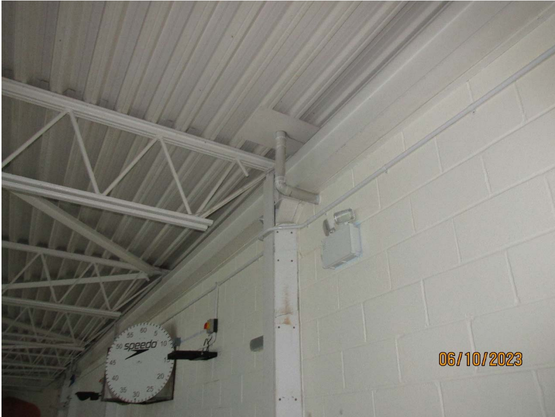
Eaves beam on steel columns supporting Lattice Roof trusses above the Swimming Pool
