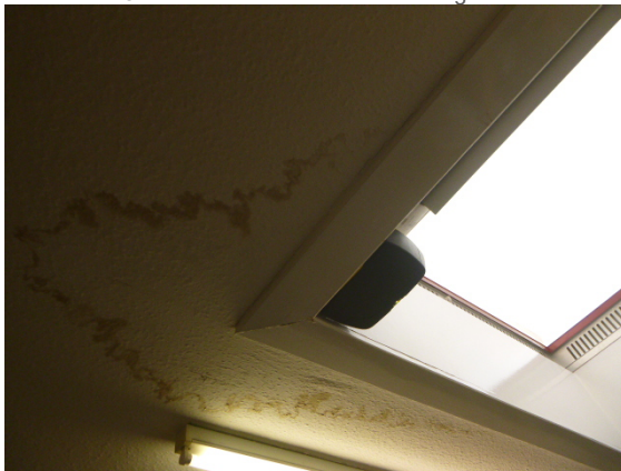
27. Staining of the office ceiling due to roof light leakage.
