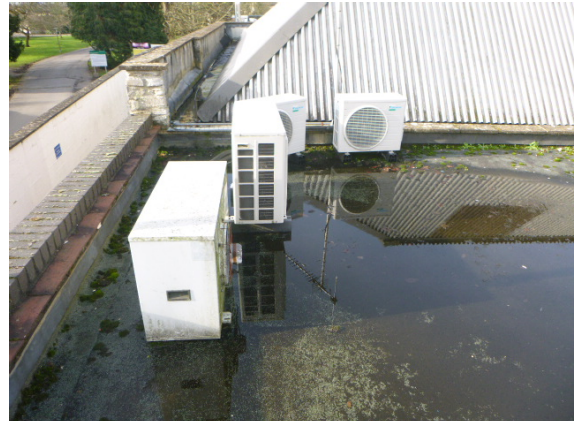
16. Standing rain water ponding to flat roofs due to poor provision of gradient will lead to accelerated breakdown.
