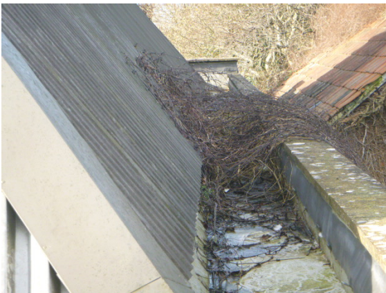
11. View of the rear parapet gutter run – heavy vegetation growing and blocking the ability of the gutter.
