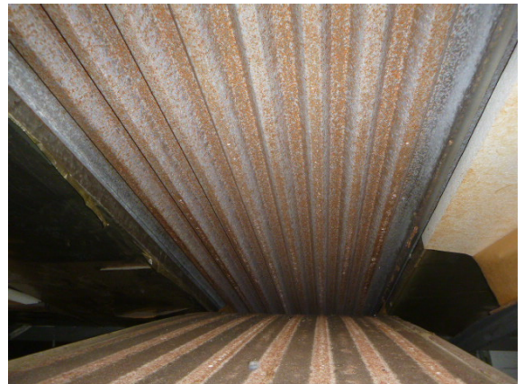
36. Loss of adhesion to the insulation panels beneath the clad roof of the assembly Hall plus corrosion due to moisture run off.
