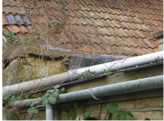
20. Roof flashing and guttering to the rear dressing room with vegetation growth blocking and slipped flashings.
