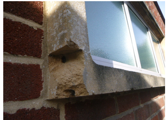
4. Spalling reconstituted stone window surround with corroding rebar.
