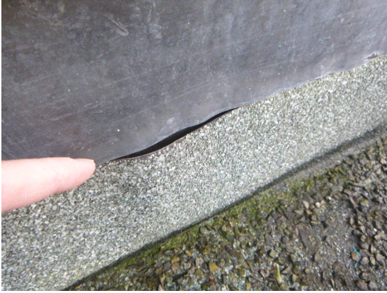
13. Typical workmanship failure of the flat roof felt upstand and lead flashing allowing rain to penetrate behind.
