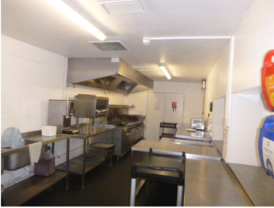
31. Kitchen facility – tenants fit-out.
