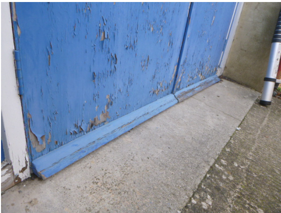
9. Side fire exit doors in poor repair.
