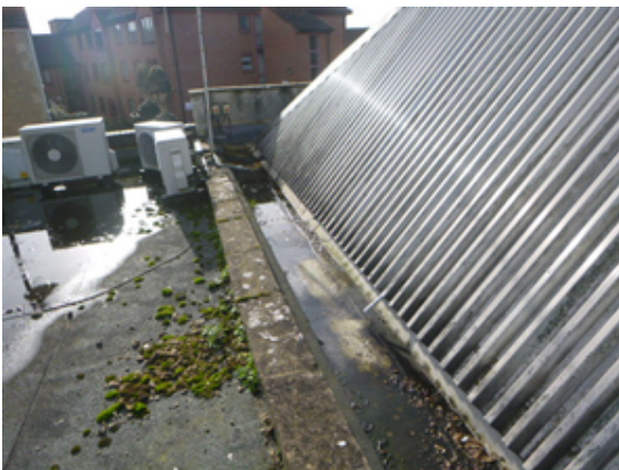
23. Metal pitched roof to the Hall, parapet gutter and loose copings.
