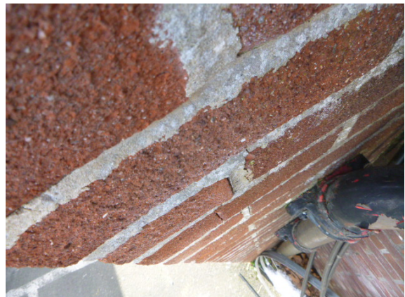
6. Expansion crack along the front elevation.
