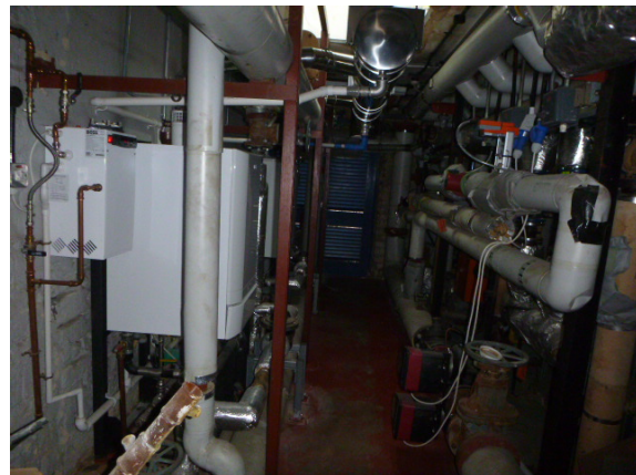
30. Main boiler room with plant for both the Assembly Hall and the Swimming Pool.
