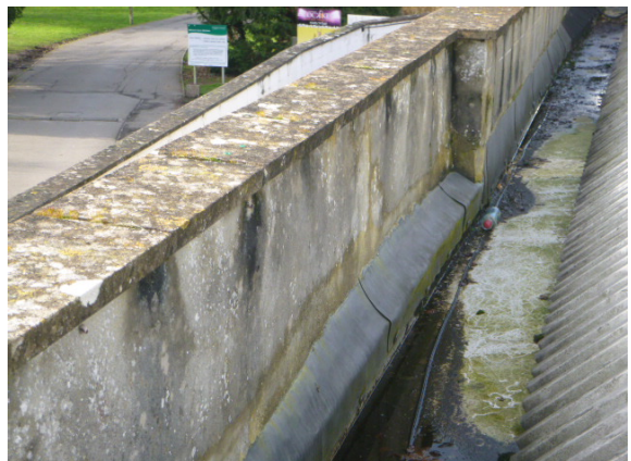
18. Crude lead flashing details and hollow render to the left side parapet. Parapet gutter noted to be offering minimal gradient. Copings lose requiring rebedding (H&S risk).
