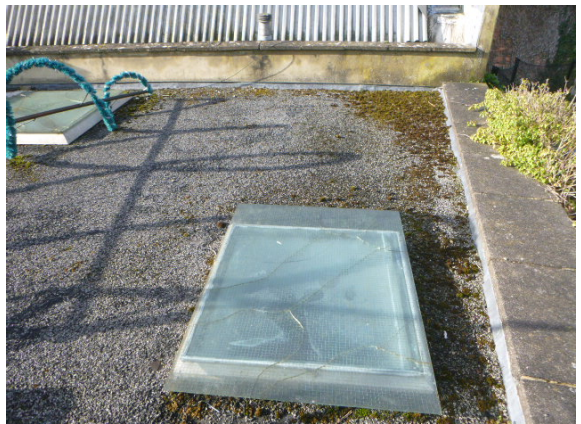
12. Cracked Georgian wired roof lights over the Dressing Rooms.
