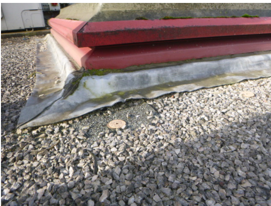
17. Lead upstands to office / foyer rooflights split and inadequately detailed reflect continuing leaks.
