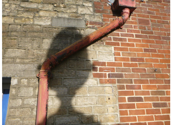
8. Brick to stone junction along the left elevation and failing décor to the cast iron downpipe hopper.
