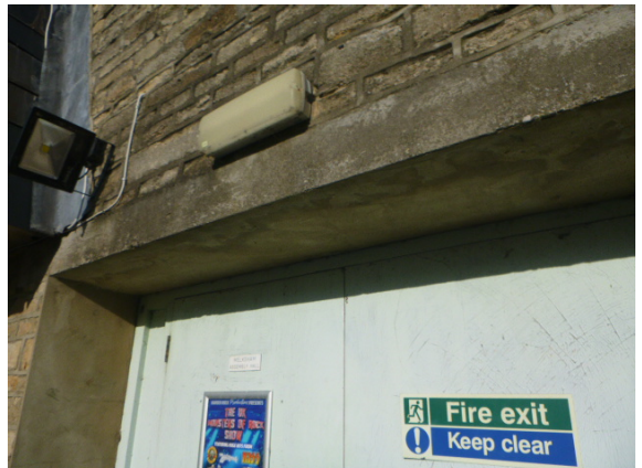
10. View of the fire exit door heads with rain tracking under the lintel and staining the finish.
