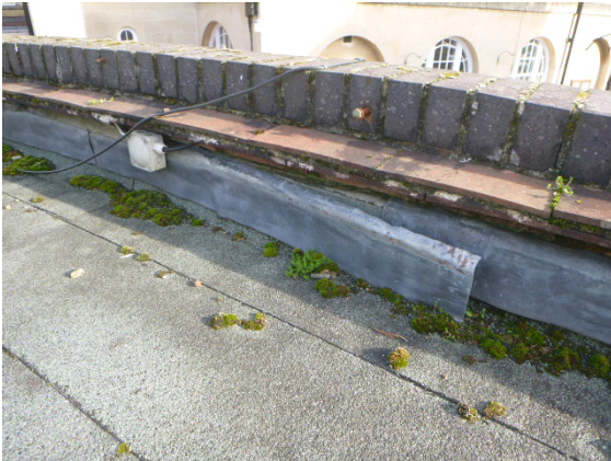
15. Slipped lead flashings to the parapet upstands. Moss accumulation.
