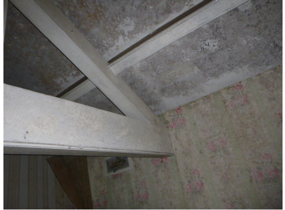
32. King post trusses embedded in the solid wall of the older section of the central core – prone to wet rot.
