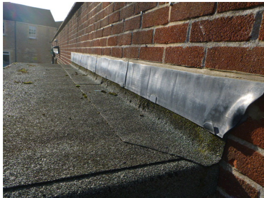
3. Lead work flashing and felt over the main front door awning canopy.
