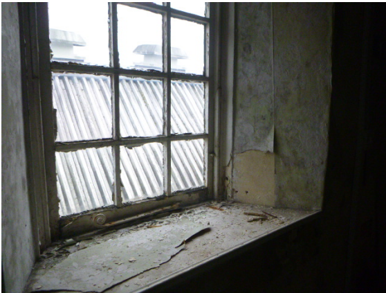
33. Typical old neglected window to the central core section upper floors. Looking towards the rear clad pitched roof slope.
